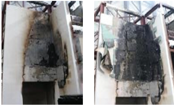
(a) Front view after test (b) Undamaged finisher Fig. 18. Fire Damage (EIFS 2)
