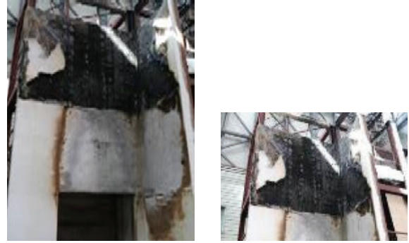
(a) Front view after test (b) Detailed view Fig. 20. Fire Damage (EIFS 3)
