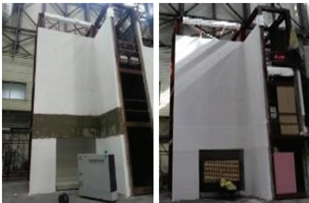
(c) Installation of Glass Fiber Mesh on Insulation (d) Finish the EIFS
