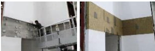
(a) Demolishment of Existing EIFS (Length: 1,000 mm) (b) Reconstruction of Insulation with Mineral Wool
