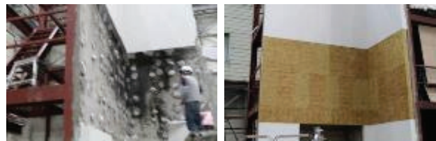
(a) Demolishment of Existing EIFS (Length: 2,500 mm) (b) Reconstruction of Insulation with Mineral Wool
