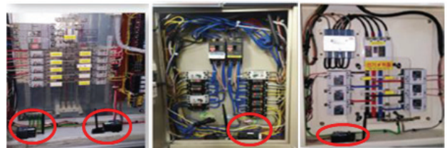
Fig. 2. Instrument Applied to the Market Distribution Board
