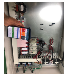
(b) Distribution Board
